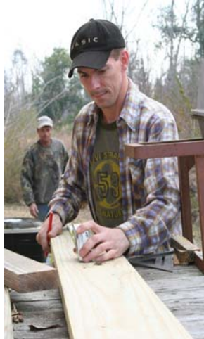
Mississippi--A carpenter trims a joist in a CWS-supported project to re-level a home that slipped off its piers during Hurricane Katrina. Photo: Matt Hackworth/CWS
