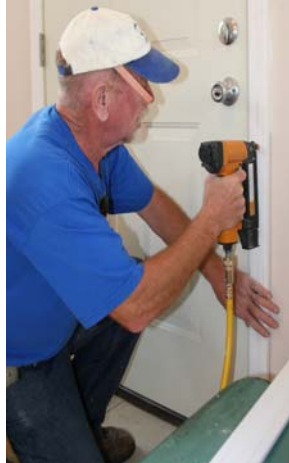
A volunteer installs a new door frame in a damaged home in Slidell, Louisiana. Photo: Matt Hackworth/CWS
